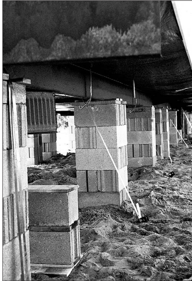
Figure 2-5. Typical installation of a manufactured home on masonry block piers with tie-down straps.
