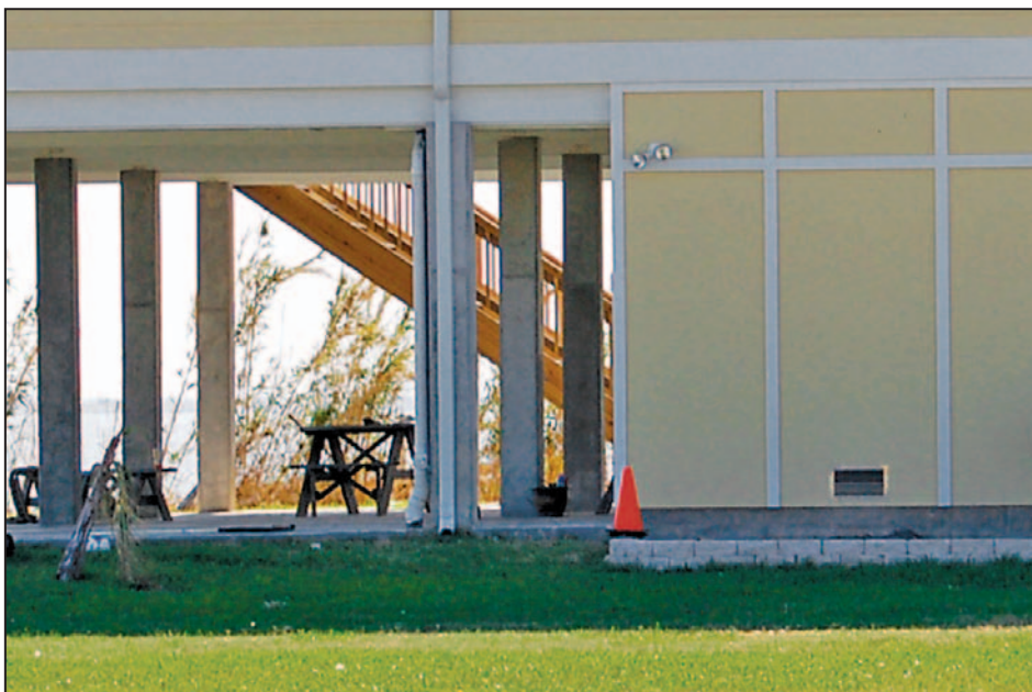
Figure 2-20. Flood opening in an enclosure with breakaway walls, Hurricane Ike (Galveston Bay shoreline, San Leon, TX)
