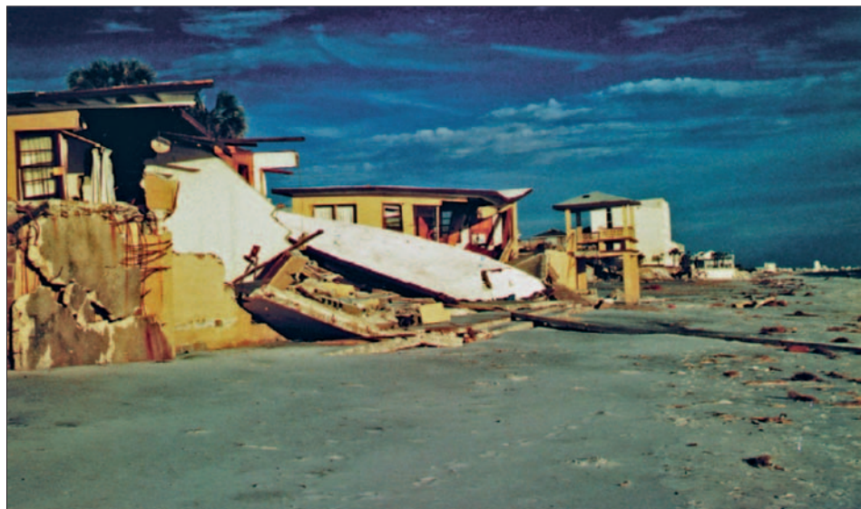
Figure 3-45. Failure of seawall in Bay County, FL, led to undermining and collapse of the building behind the wall (Hurricane Opal, 1995)
