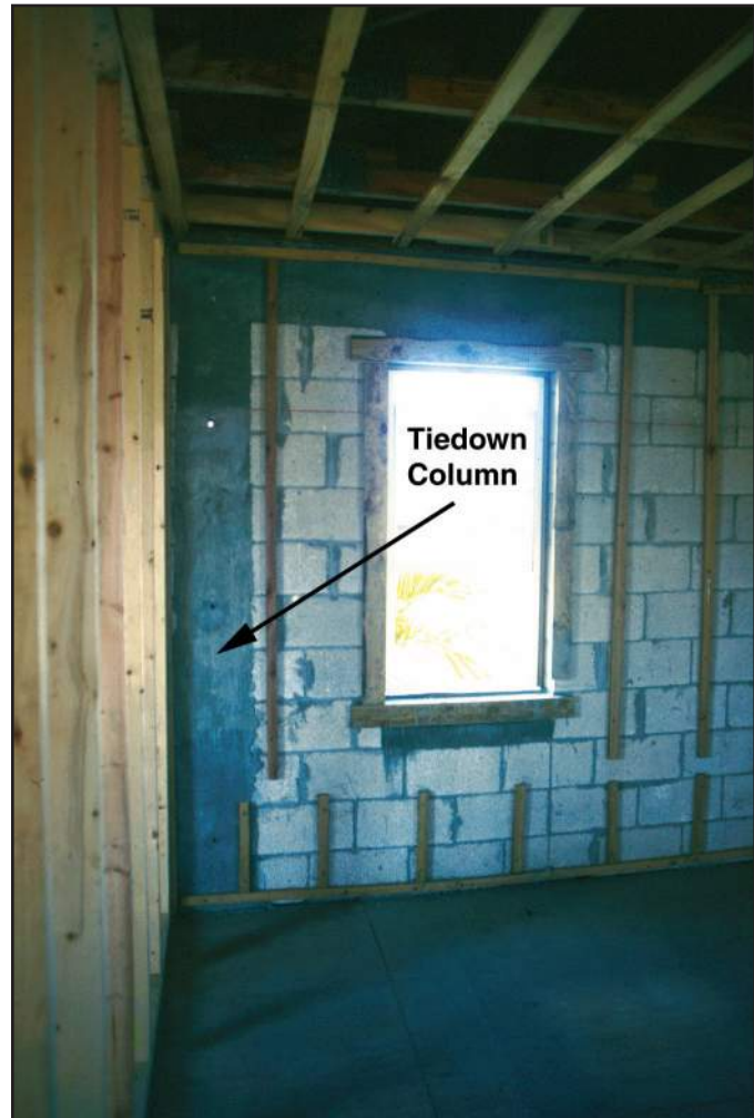
Figure 46 Concrete tiedown columns, such as the one to the left of the window in this photograph, were also used in this house.
