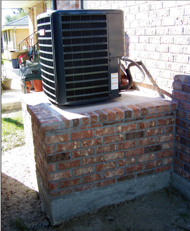
Figure 3-1. Air conditioning compressor elevated on a pedestal.
